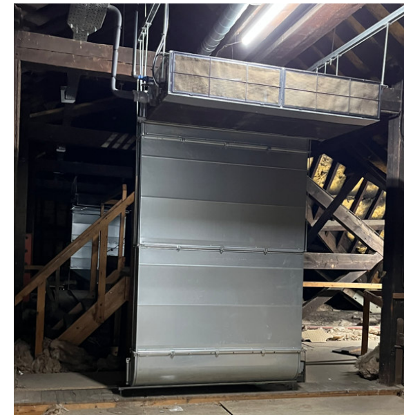
Ducted heating and cooling units to Victoria rooms within loft space, provided by fresh air by local fans. Unit over large venue/conference space.
