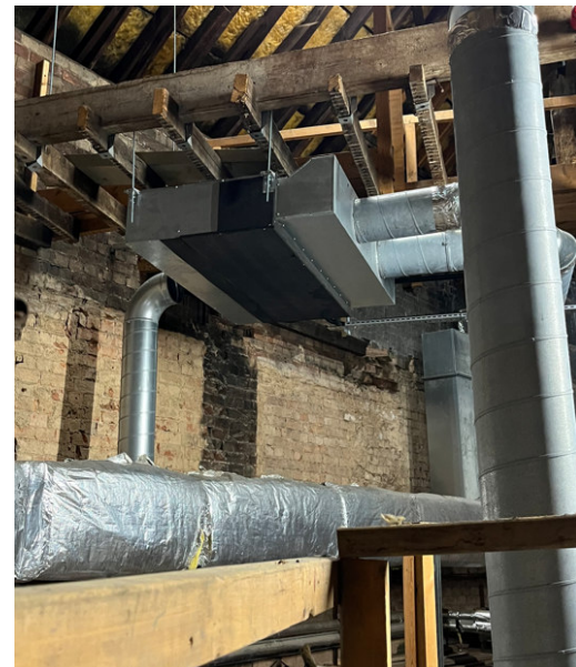
Ducted heating and cooling units to Victoria rooms within loft space, provided by fresh air by local fans. Unit over bar space.
