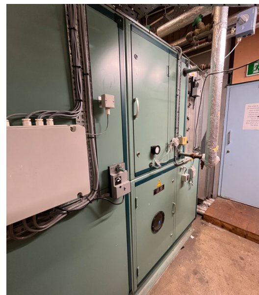
AHU02 serving function room in mezzanine plant room.
