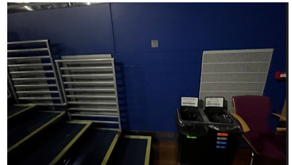
Performance hall ventilation grilled run along either side wall of the hall itself in the form of sidewall grilles providing ventilation, with heating and cooling provided by treating the incoming air. Air delivered below the bleacher seating.
