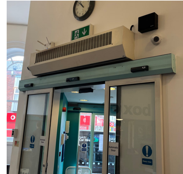
Overdoor Air Curtain to entrance draught lobby.
