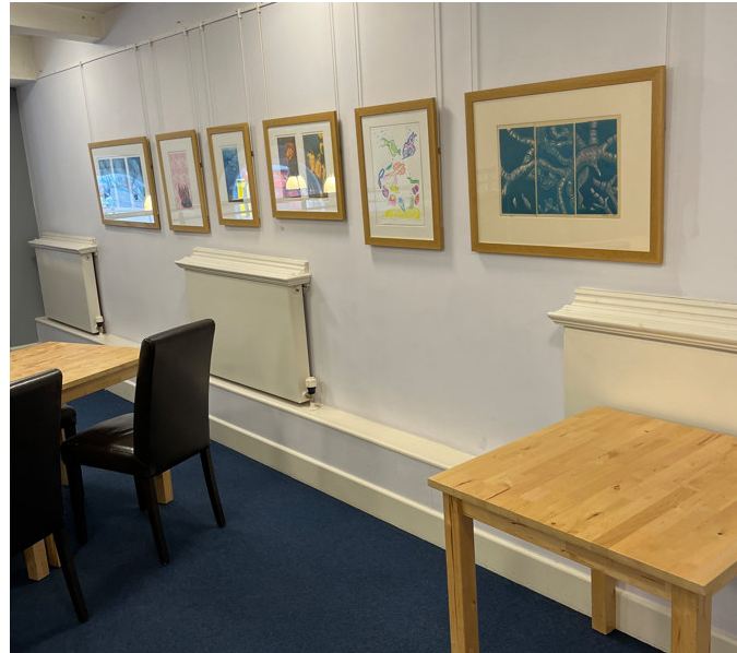
General Heating Installations – Aged Radiator heating via gas fired boilers.
