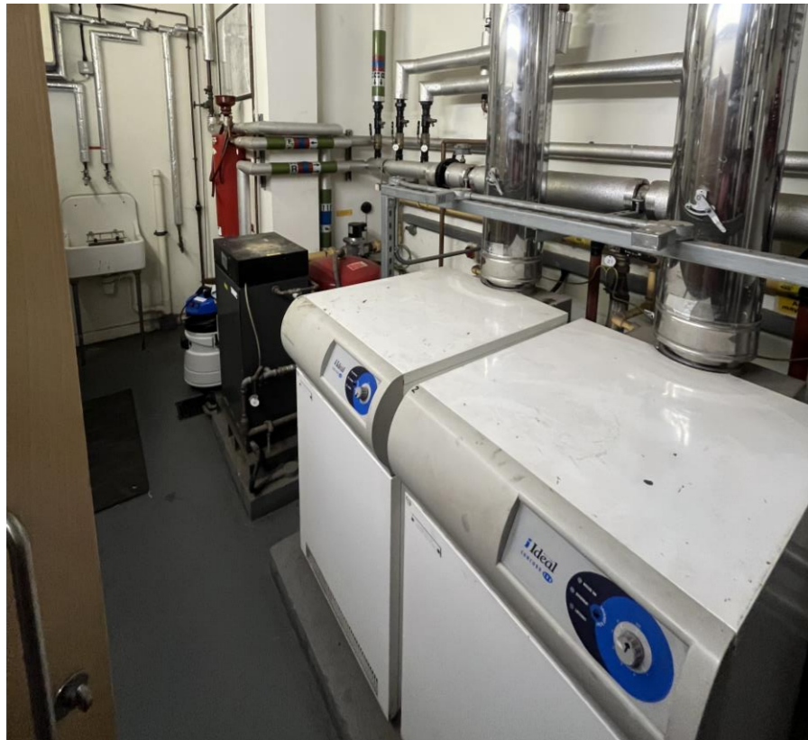
Existing Gas Fired Boilers
