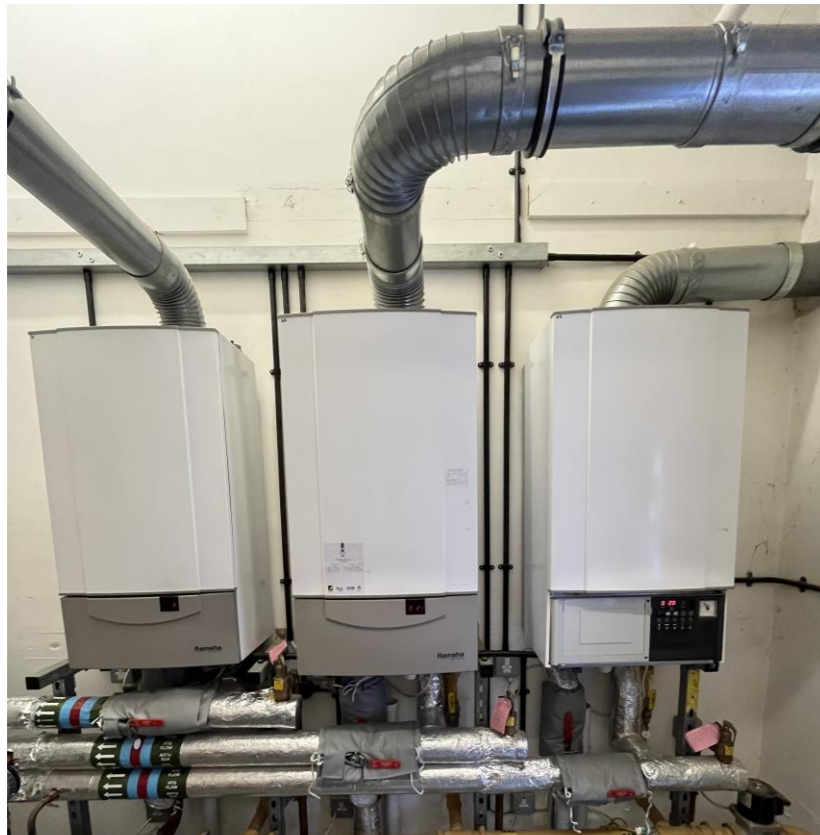
Existing Gas Fired Boilers
